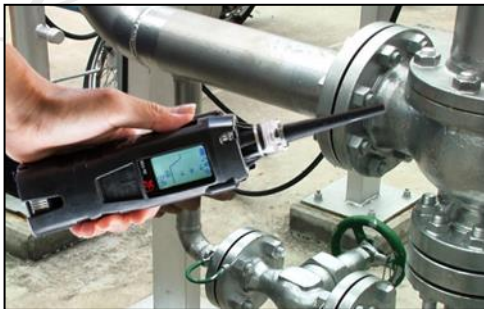
For gas pipe joint
